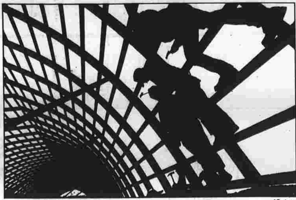
BARN FRAME - Neighbors and friends work on the beams of a new barn under construction at the Lyndon Corey farm in Fairfield, Vt. last week. Corey lost his barn and some livestock to a fire this winter. The new barn will measure 212 feet by 40 feet and will house 100 cows.
